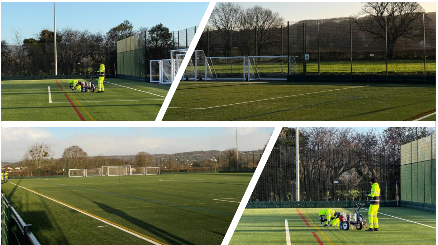
The above slide shows the finishing touches to the 3G pitch just before the Christmas break.
